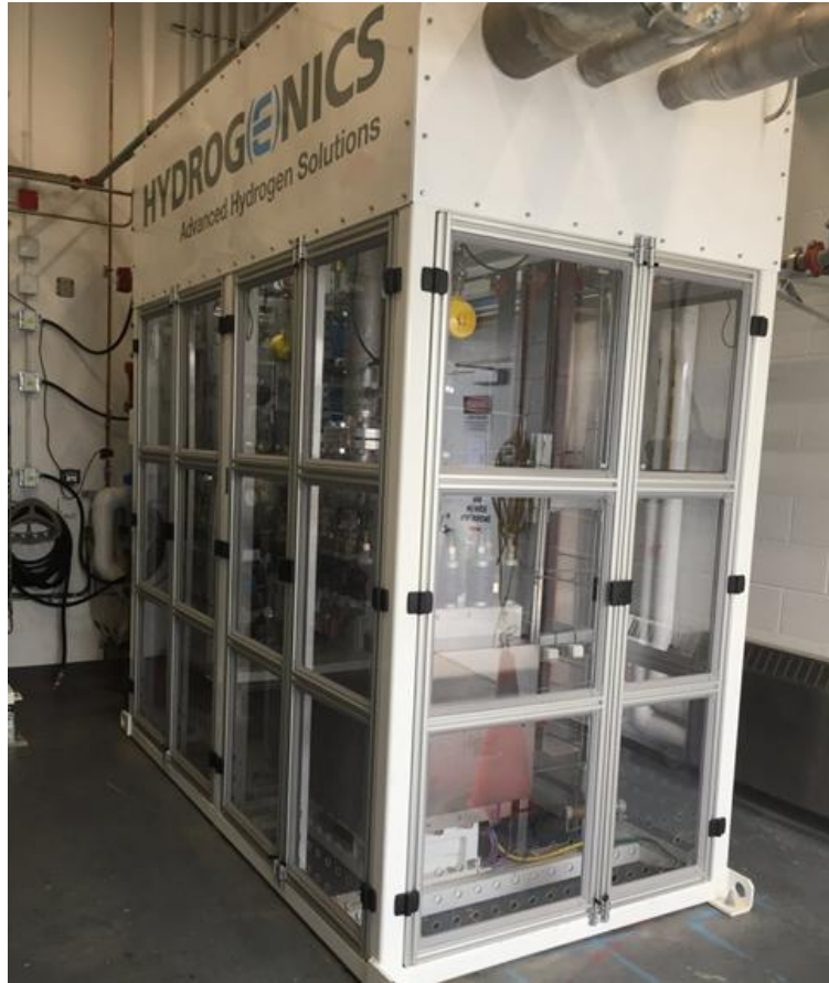
North America's first Power-to-Gas energy storage
